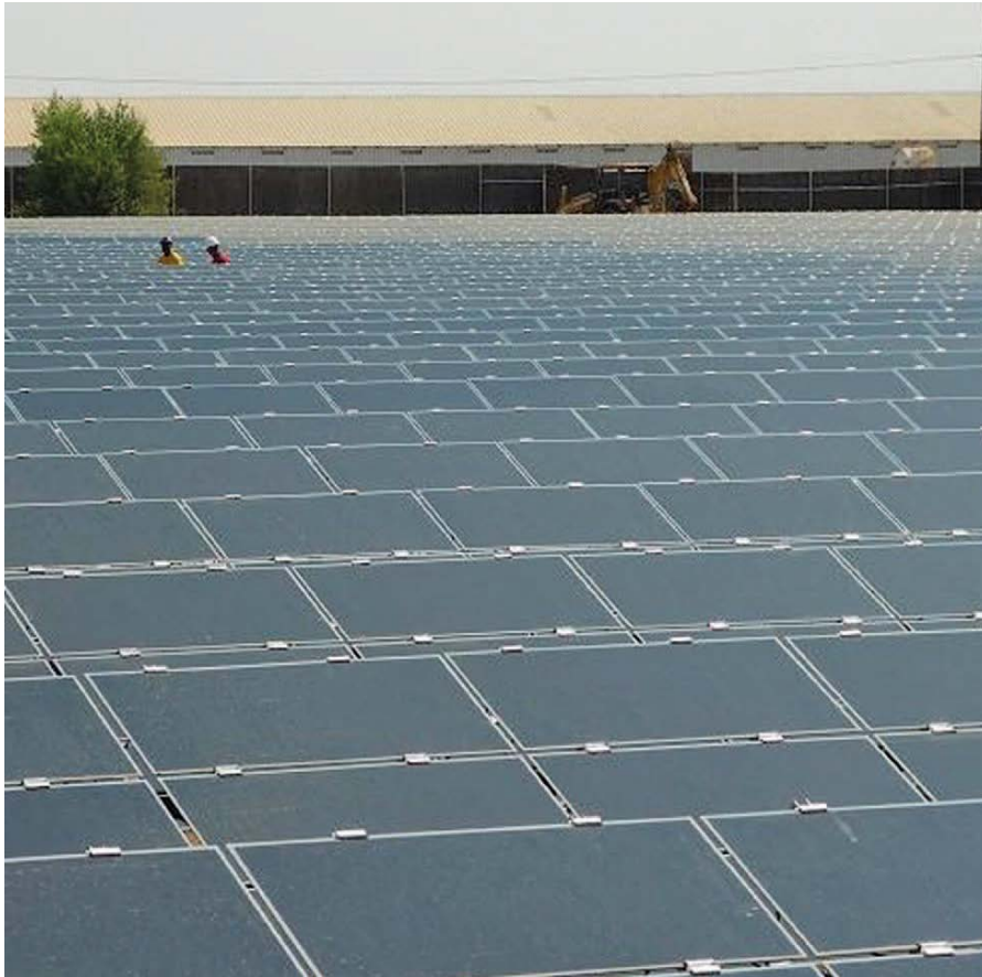
Photo from SMUD's SolarShares Installation
